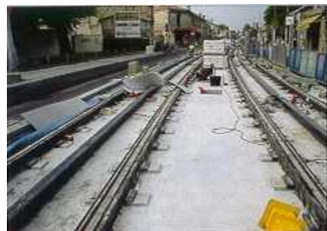
A third rail section nearing completion near the University of Talence (CJ Wansbeek)
